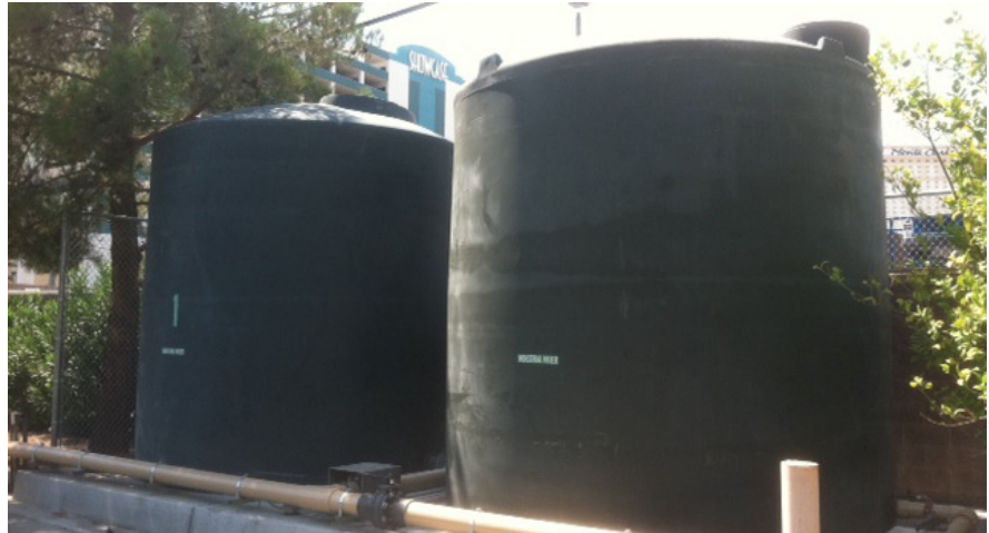
Well Tanks Close Up
